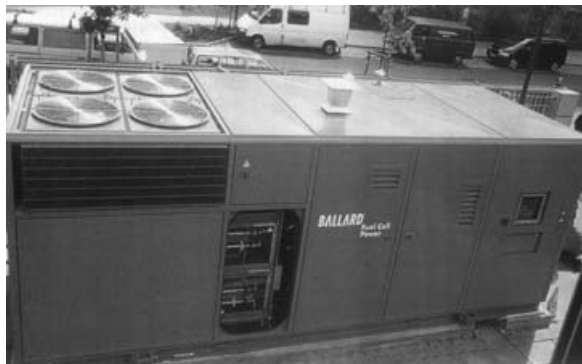
Figure 11: 250 kW fuel cell charged by natural gas
