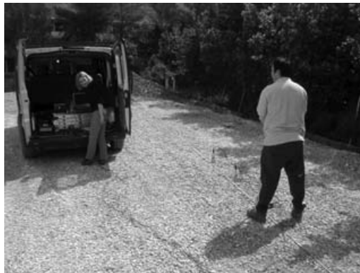
Figure 8: Quality control of soil improvement by the Spectral Analysis of Surface Waves method
